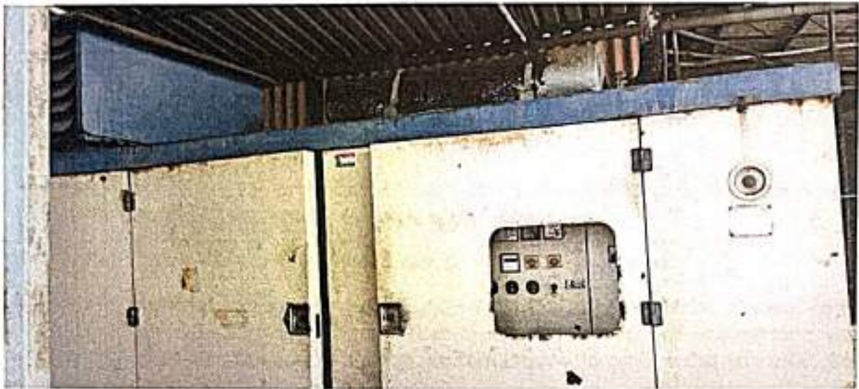
Photo-2: DG set up at Siddhant College of Pharmacy, campus Pune
