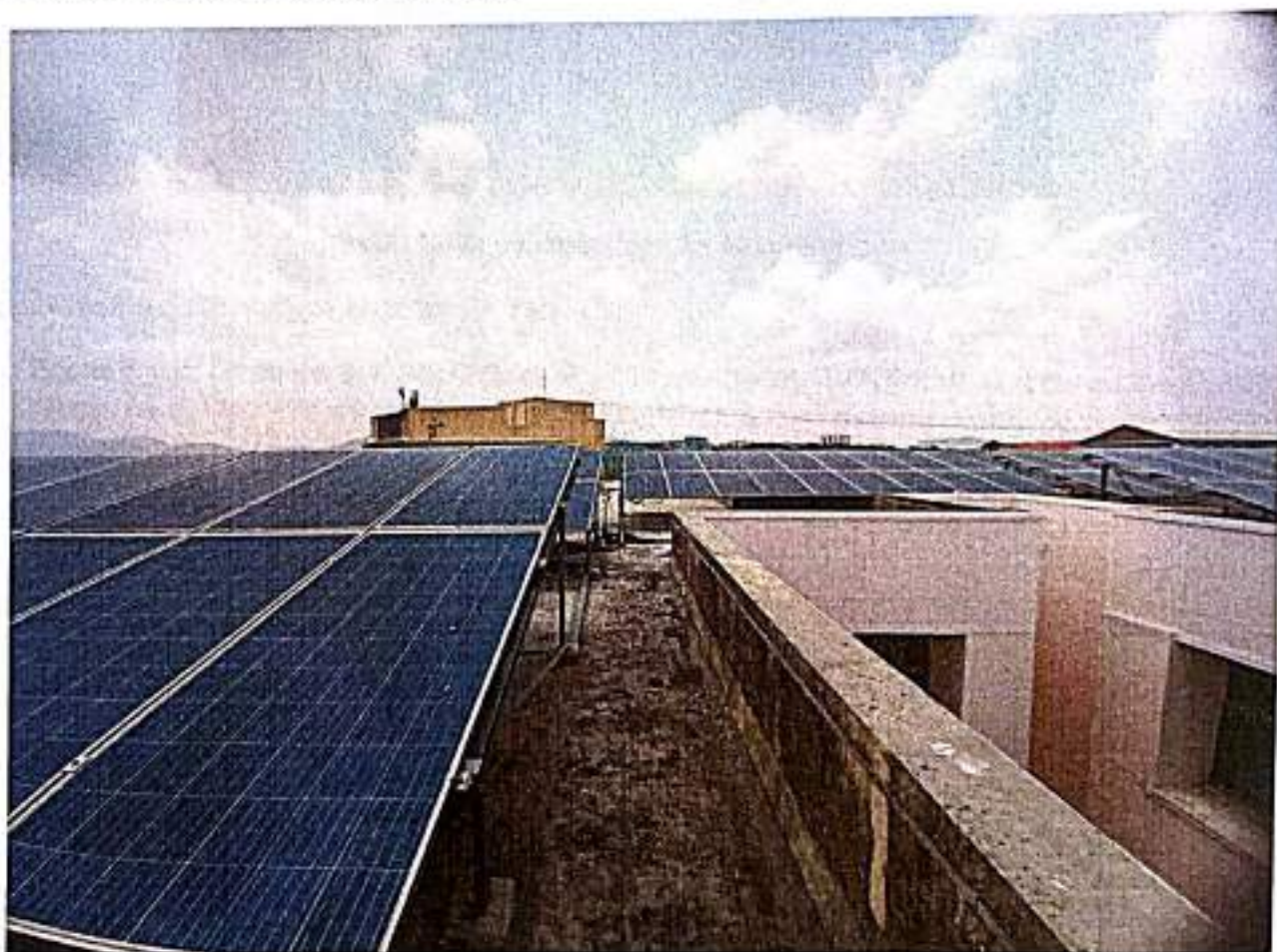
Photo-5: 221 kW solar roof top on Siddhant College of Pharmacy building roof.
