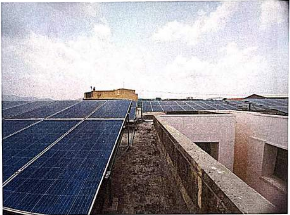
Photo-1: 221 kW solar roof top on Siddhant Pharmacy college building roof.
