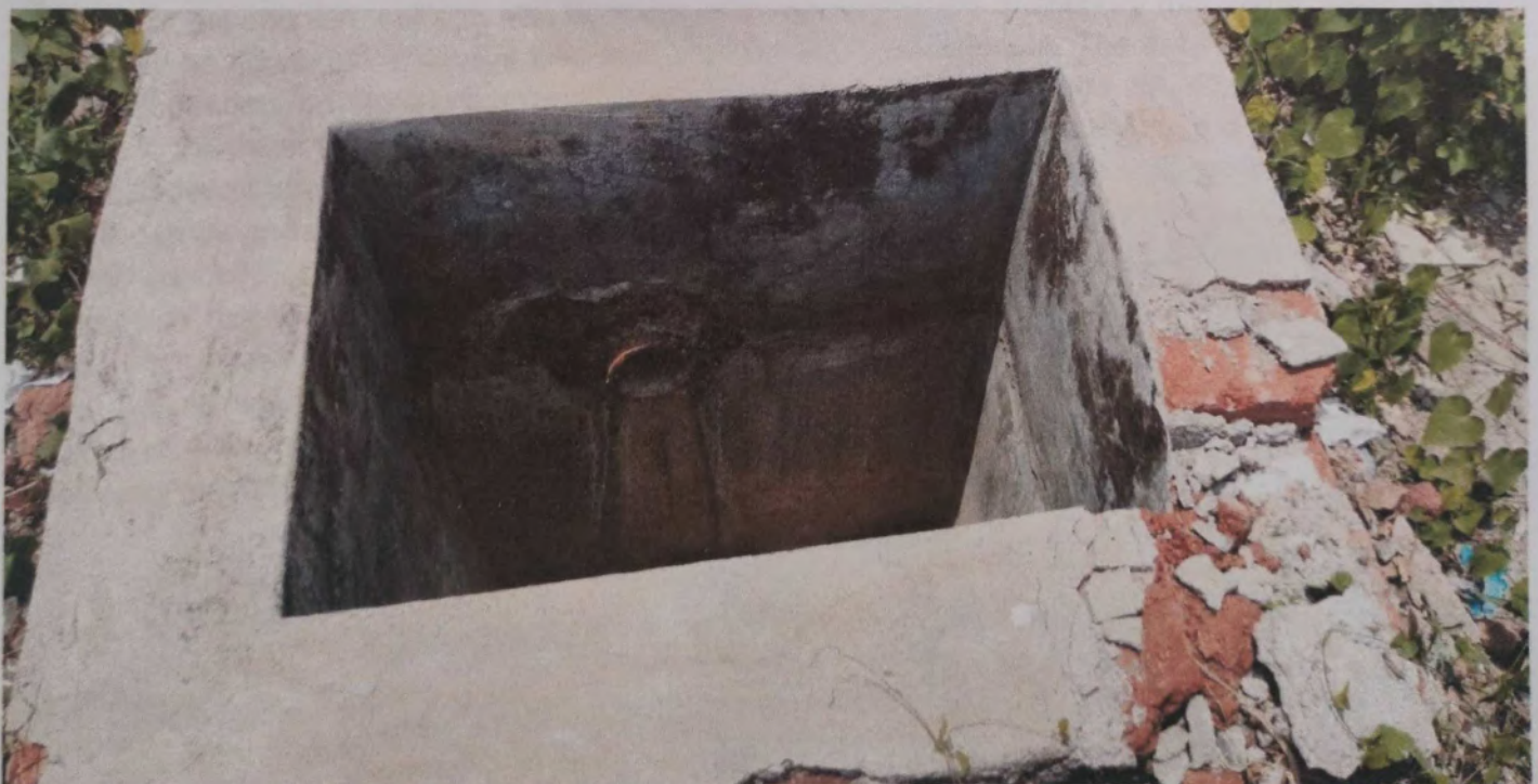
Photo-6: View rain water collection from building
