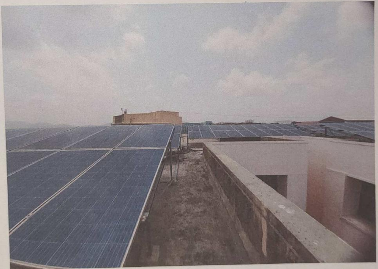
Photo-5: 221 kW solar roof top on Siddhant College of Pharmacy building roof.
