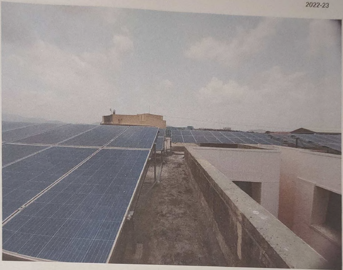
Photo-1: 221 kW solar roof top on Siddhant Pharmacy college building roof.
