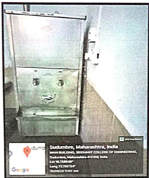
Water cooler for drinking water
