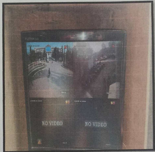
CCTV Surveillance system
